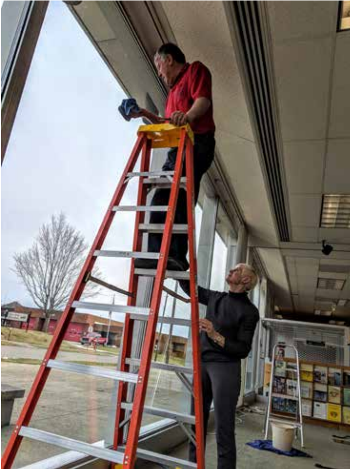
After the new blinds were installed, the inside of the windows had to be cleaned before the gift shop cases could be moved back in place. Joe and Sharon Miller know just how dirty the windows were!
