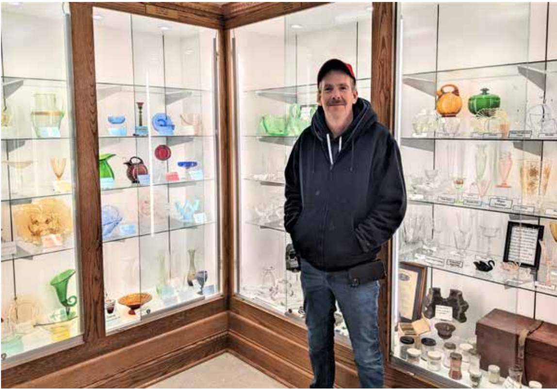
The Museum electrician, Ben Kirkman, installed the new LED top lights in each case in the Education Center. These cases never had any puck lights so it made quite a difference!
